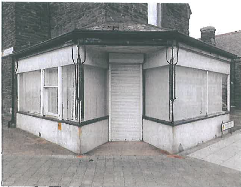
Plate 22 – Corner of south west and north west elevation. Retail unit facade noting shallow roof pitch, general condition and corroded condition of metalwork for the shopfront awning
