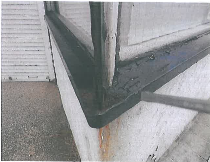
Plate 26 – North west elevation retail unit, noting poor condition of the timber window sill section
