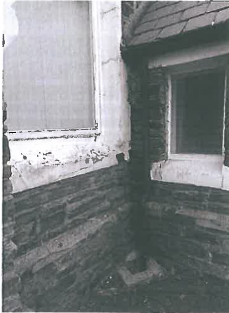
Plate 13 – South west elevation external wall thickening at low level with concrete capping detail, noting general condition of the concrete capping to the wall at low level, cracked and crazed render to the window surround and poor condition of the render to the window head detail
