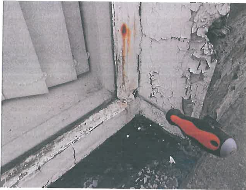
Plate 27 – North west elevation, retail unit, noting poor condition of window to the W.C.
