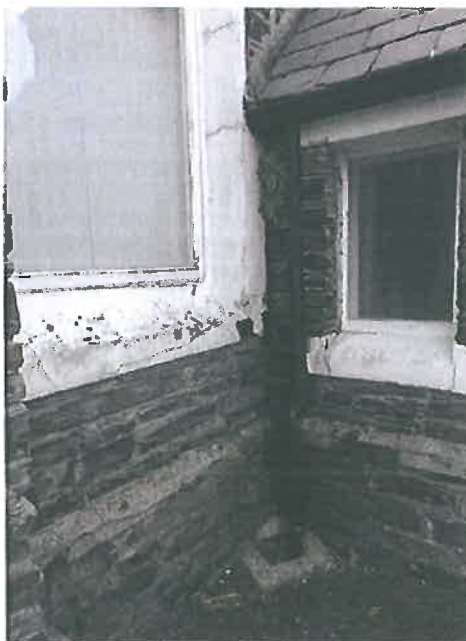
Plate 14 – South west elevation, south porch noting vegetation and damp staining to the wall. Note general condition of the concrete capping to the wall at low level and the concrete window surrounds
