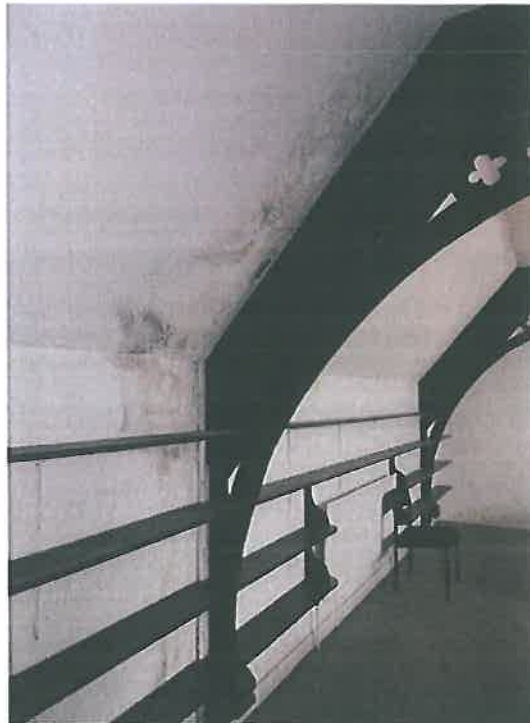
Plate 48 – First floor office (south) noting damp ingress to wall and roof around decorative principal truss
