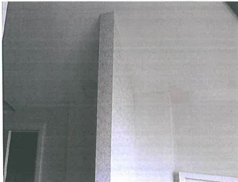
Plate 56 – Residential unit bathroom noting damp ingress to the wall and soffit
