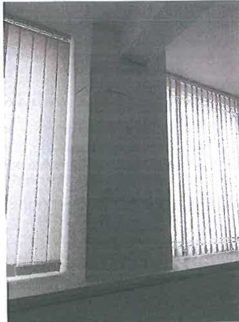
Plate 40 – Office, external wall noting damp ingress
