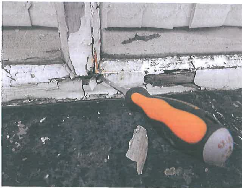
Plate 28 – Window, noting poor condition generally
