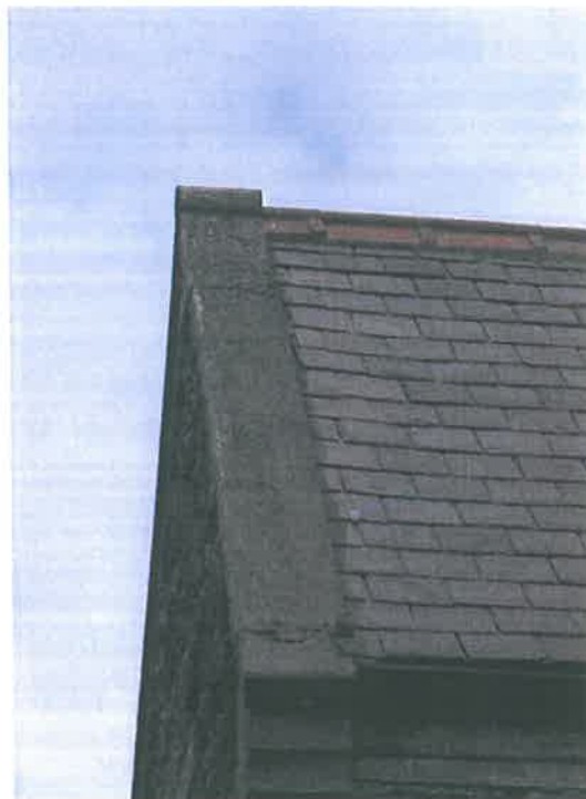
Plate 8 – Residential unit roof verge capping, noting cracking to the capping
