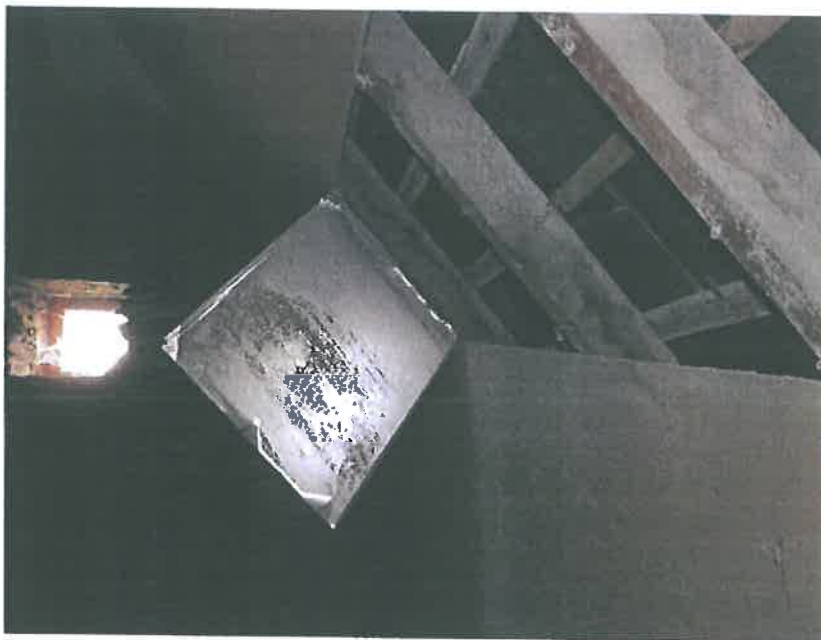
Plate 54 – Residential unit, north roof void noting rafters boarded with foil backed plasterboard and damp staining to rafters
