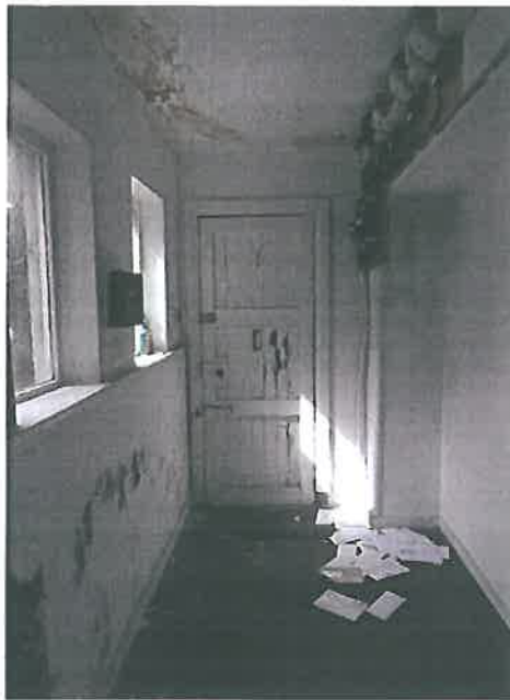
Plate 31 – North porch interior noting general condition and multiple meters and electrical equipment
