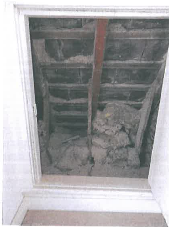
Plate 53 – Residential unit, second floor, eaves void cupboard noting lack of torching and general condition
