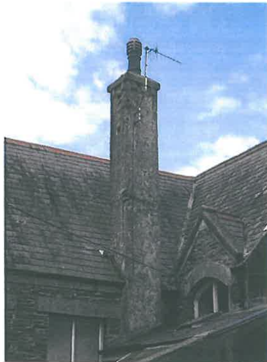
Plate 10 – Chimney stack between Manxonia House and Overcliff, noting poor condition of the render and vegetation and lichen growth evident to the top of the stack and at the roof junction.
