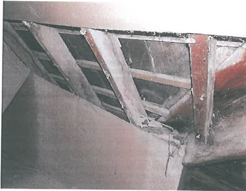
Plate 57 – Residential unit, north roof void, noting damp staining to the valley lay board and rafters
