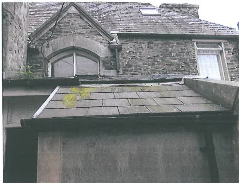
Plate 12 – Mono pitch roof to the kitchen noting manmade slate and general condition
