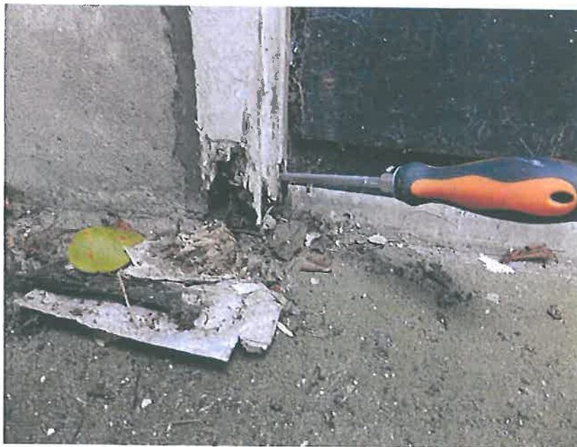
Plate 30 – North east elevation, kitchen door, noting rot to the door frame and general condition
