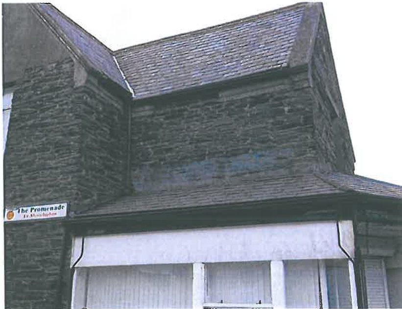
Plate 16 – North west elevation, noting painted section of wall above the retail unit roof
