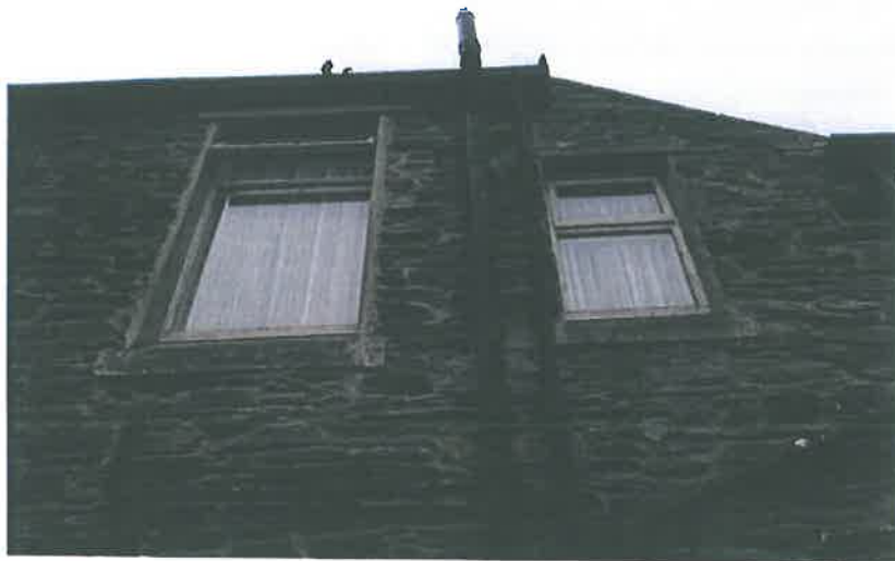
Plate 18 – North east elevation noting vegetation to the gutter, cracked concrete to the window sills, patched/pointed stone and general condition of window
