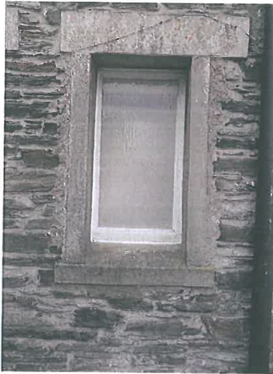
Plate 29 – Window to the retail unit noting poorly applied mortar around reveal detailing
