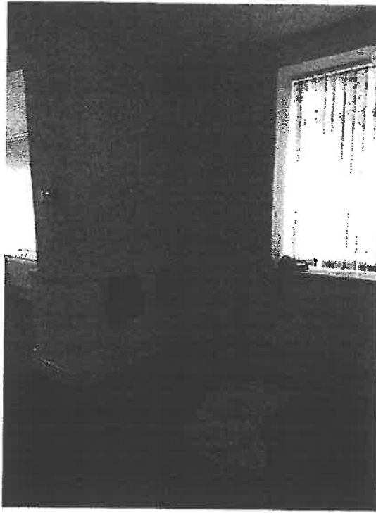
Plate 43 – Retail area, damp ingress to walls
