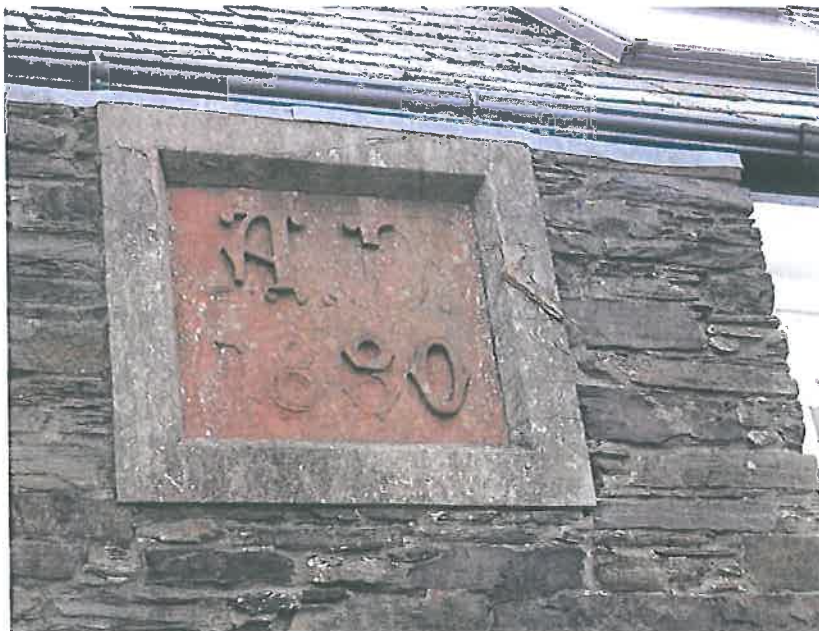
Plate 20 – South west elevation, noting the lead capping to the external wall and deterioration of the sandstone plaque
