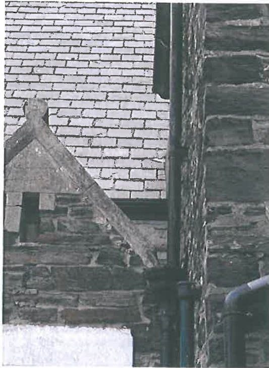
Plate 21 – South west elevation, south porch apex to gable noting crazed and cracked concrete areas, missing facing to apex porthole and areas of poor pointing
