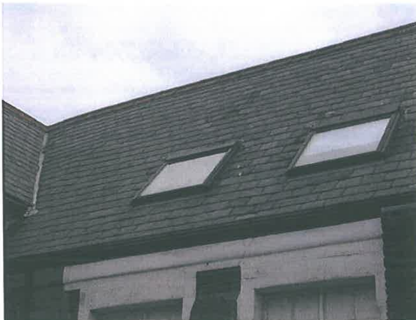
Plate 4 – Roof, south west slope noting tangles, slate chips and slipped slates to the valley. Note crazed and cracked render to the window concrete surround and head of wall detailing.
