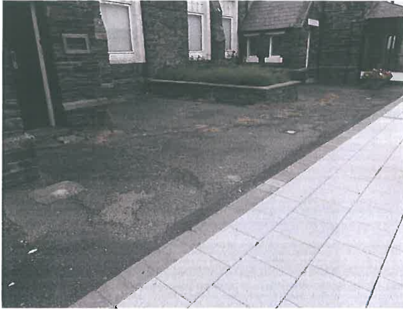
Plate 23 – South west elevation paved area, noting poor condition of the tarmac surface
