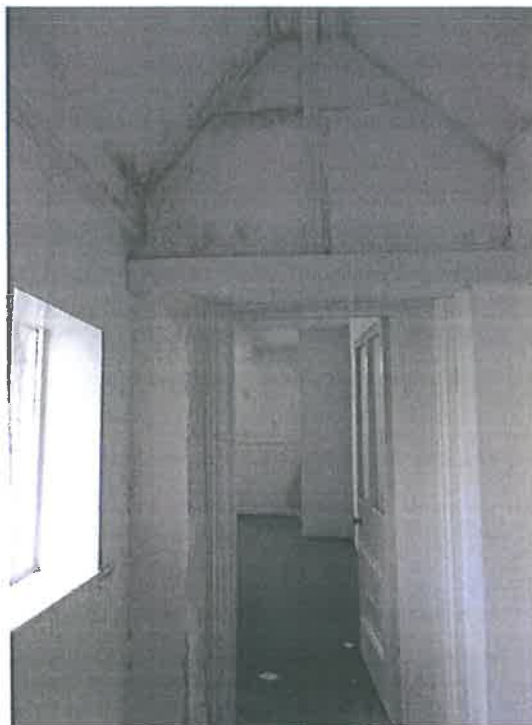
Plate 36 – South porch junction with main external wall, noting general condition
