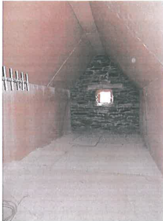
Plate 55 – Residential unit, west roof void, noting damp staining to plasterboard adjacent to the external wall and to the junction of the vertical board and sloping roof. Note build up of pointing to the floor adjacent to the wall
