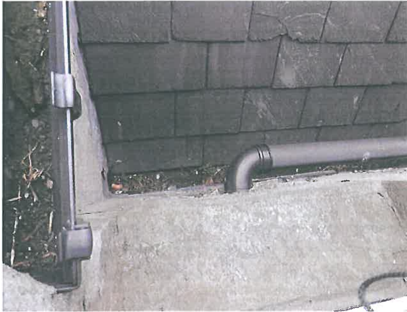
Plate 19 – South west elevation, north porch roof valley noting debris and silt to the valley and gutter to the main roof. The pipe within the valley would appear to be the soil waste from the W.C. for the residential unit
