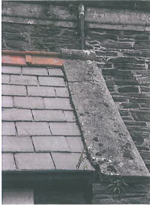
Plate 15 – South west elevation, south porch, noting cracked concrete verge detail to the roof
