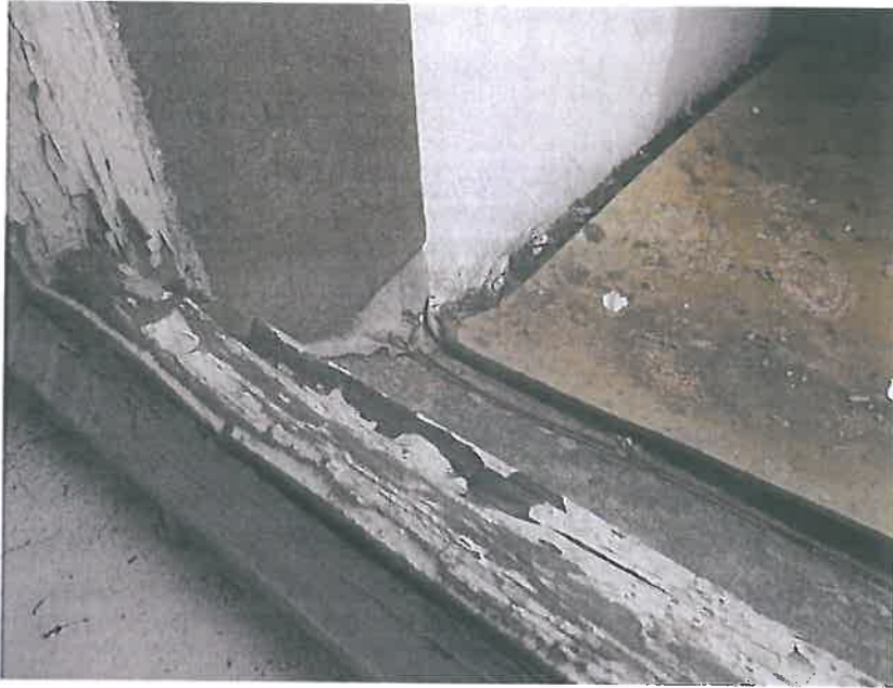
Plate 25 – North east elevation, noting poor condition of timber to window externally
