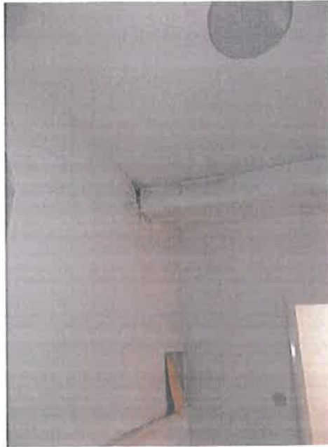
Plate 39 – Office corridor area noting damp ingress to downstand beam and external wall
