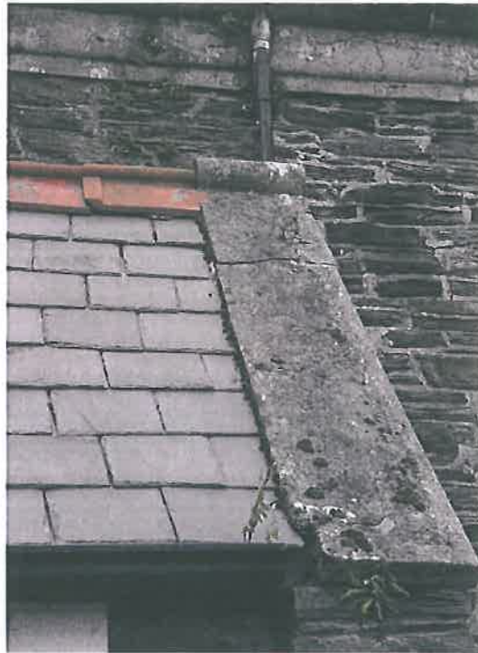
Plate 7 – Porch (south), cracked verge capping and vegetation growth
